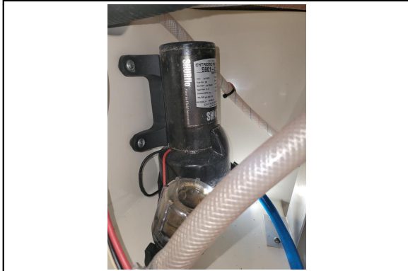
Fresh Water Pump
