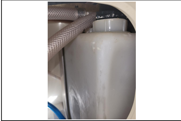
Fresh Water Tank
