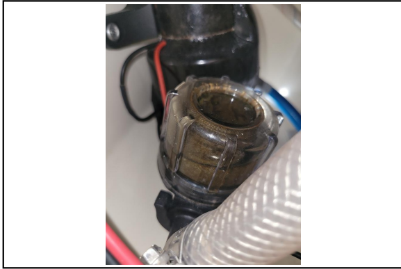
Fresh Water Filter, DIRTY
