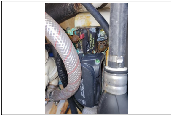
Electrical Relay CORRODED
