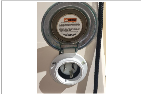
Shore Power Outlet
