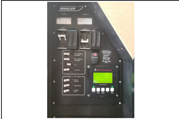
AC Control Panel
