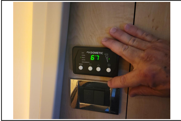
Air Condition Control
