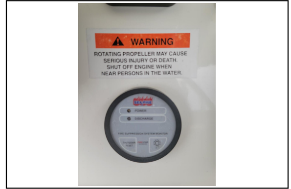
Fire Extinguisher Helm Control
