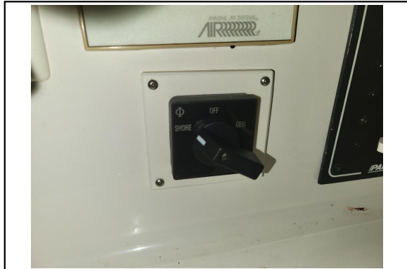
Shore Power Switch
