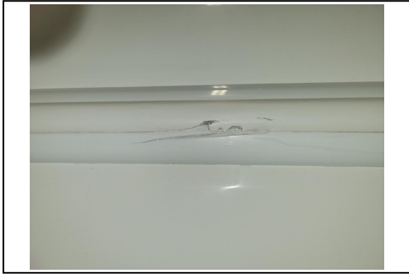
Rub Rail Insert Damage-STBD Side
