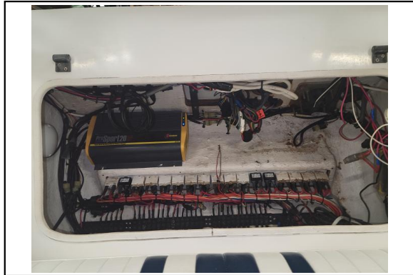
Electrical Switch Wiring, Charger
