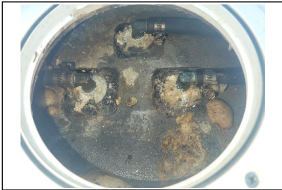
Gas Tank fittings-Corrision
