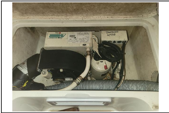
AC Unit pic 2
