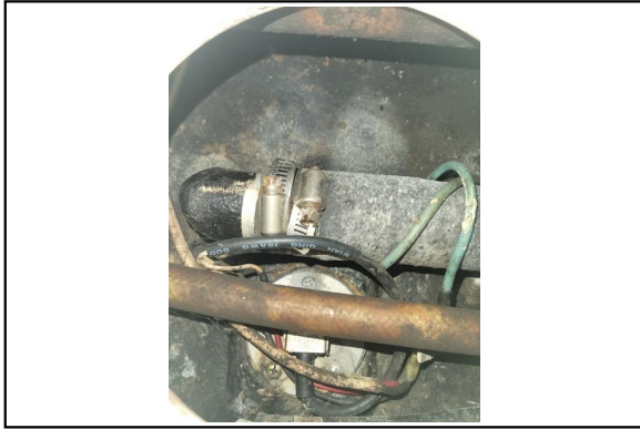
Gas Tank grounded & doubled clamped
