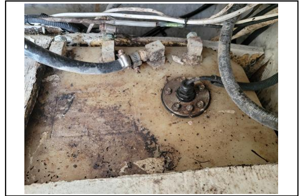
Gas Tank (Port Hull)
