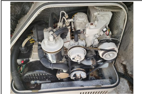
Generator, Next Gen
