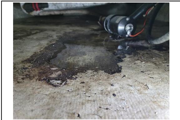
Fresh Water Pump
