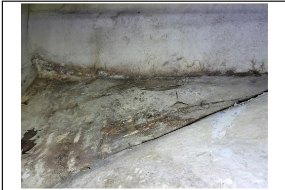
Gelco delamination in Bow Compartment
