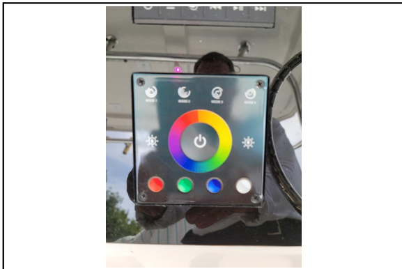
Panel Lights Control
