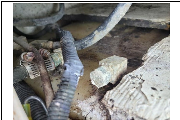
Gas Tank Fittings (STBD)
