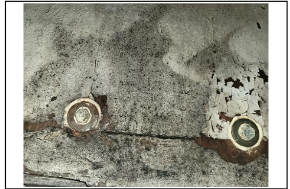
Engine Bolts- STBD Engine
