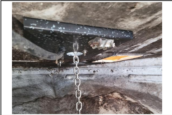
Support Board underneath Winch
