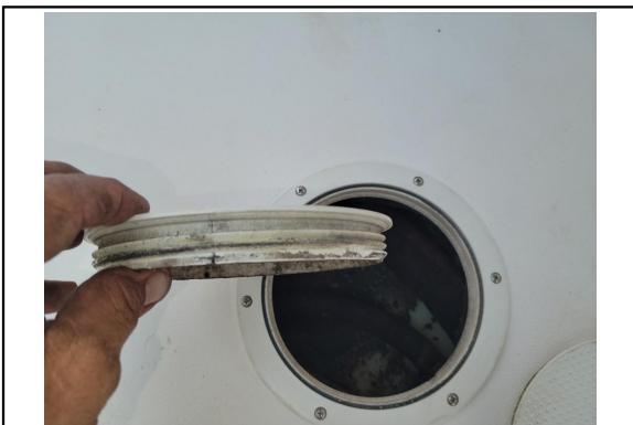
Gas Tank Deck Plates (4)
